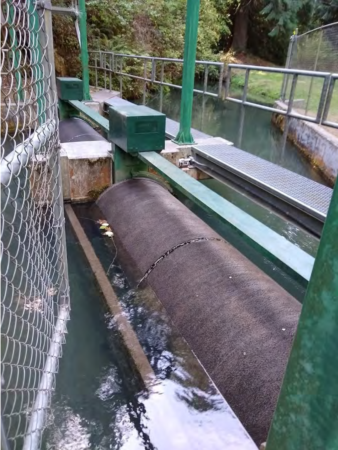
Figure 6 Two fish screens looking upstream
