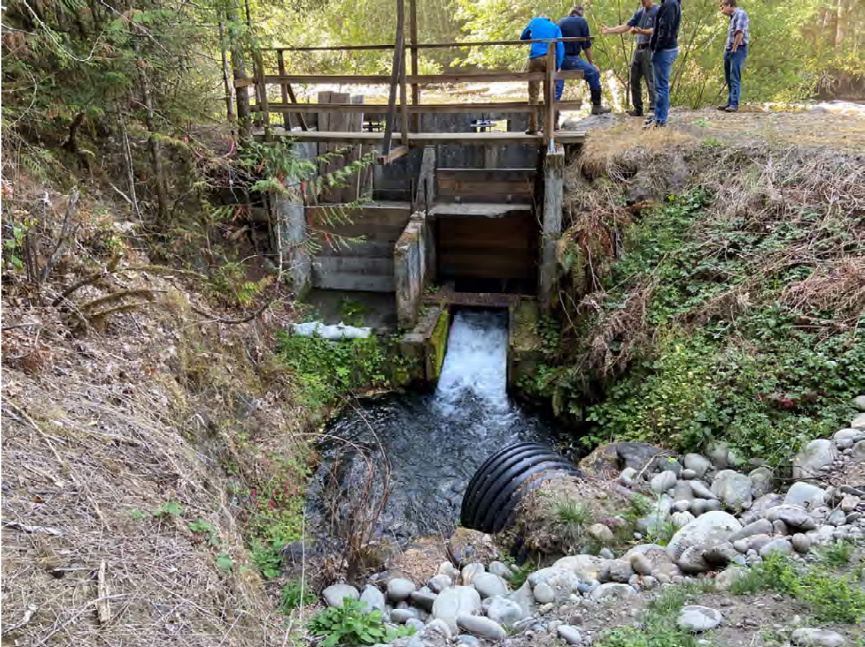
Figure 3 Highland Ditch Diversion Headgate (Two - 3 ft wide by 3 ft tall unseating head mounted slide gates)
