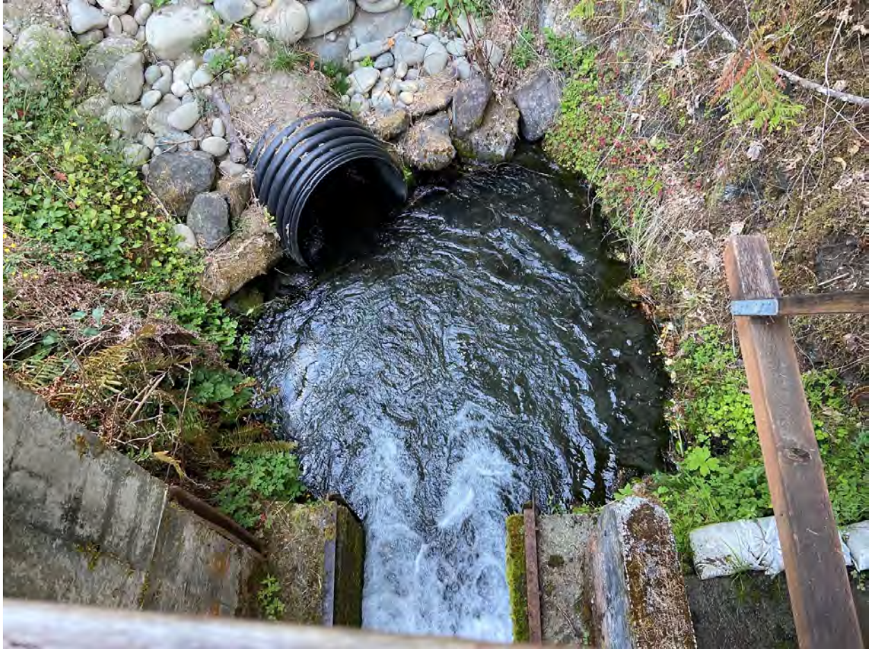
Figure 4 Highland Ditch Canal flowing through a circular ABS Culvert Pipe
