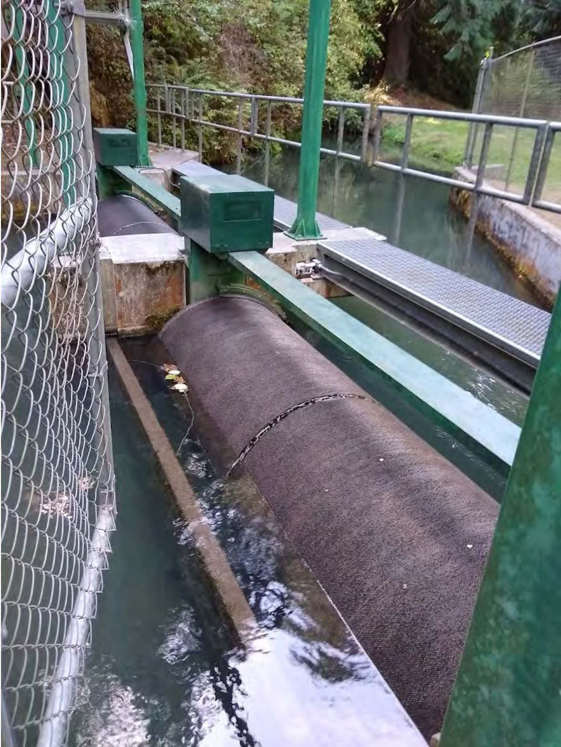
Figure 6 Two fish screens looking upstream
