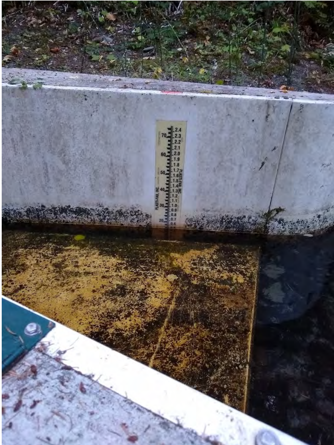
Figure 8 Parshall Flume with water depth measurement at 0.5 feet
