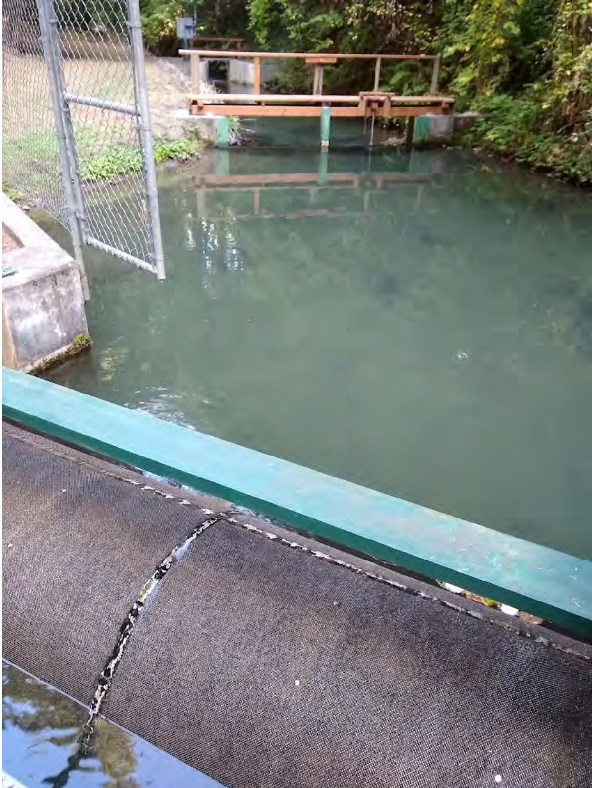
Figure 7 Stop log structure, overshoot gate and Parshall Flume downstream of fish screen
